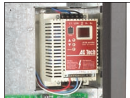
variable speed motor drive
